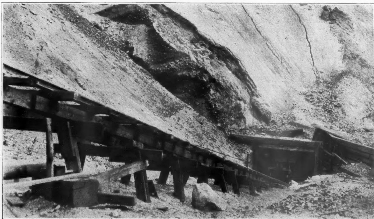
Track for Dump Car from Hopper to Crusher at Cloutier and Company
